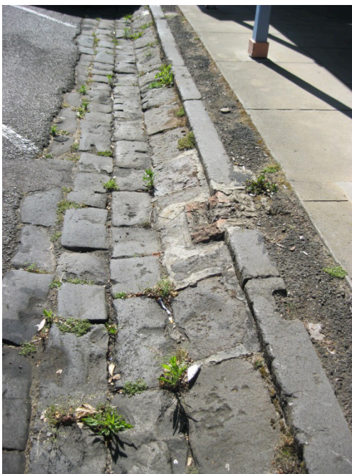
Example of bluestone gutters and the base of an original verandah post, outside 19-21 Julia Street
