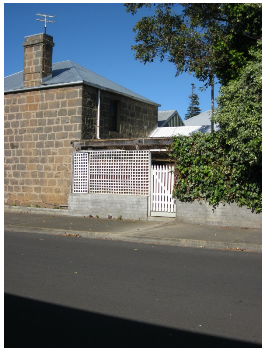
Eastern side of 16 Gawler Street, showing neat bluestone construction and chimney (significant)
