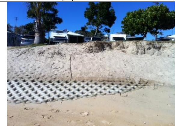
8. If vegetation is not protected and allowed to capture sand hard solutions may be required.
